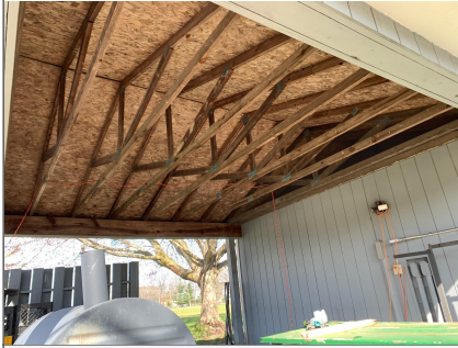
Covered back porch area, no ceiling (exposed roof trusses open to attic)
