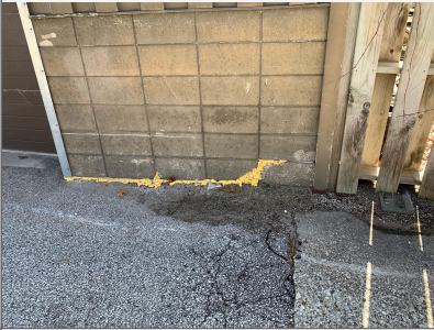
Spray foam leaking out of CMU
