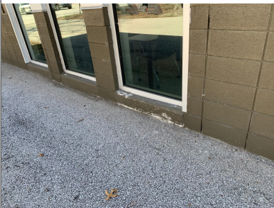
Solid concrete sills under windows (no weeps or flashing)
