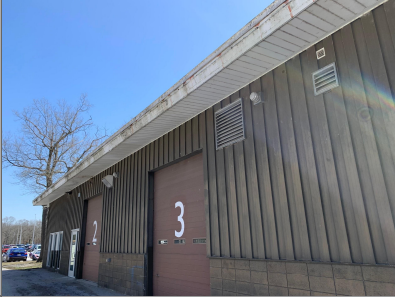
Stained fascia & soffit from lack of gutters
